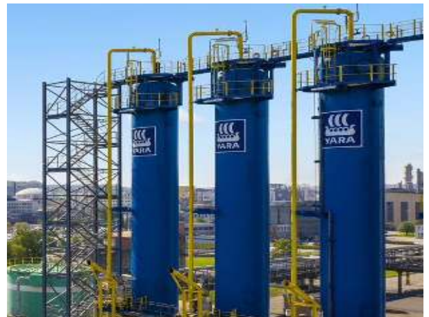
The green hydrogen demonstration plant will be the second 24-megawatt platinum-based electrolysis facility designed and constructed by Linde Engineering. Picture credit: Yara
